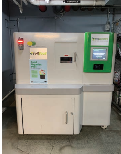
▲ The dehydrator machine at Spring Street Towers
